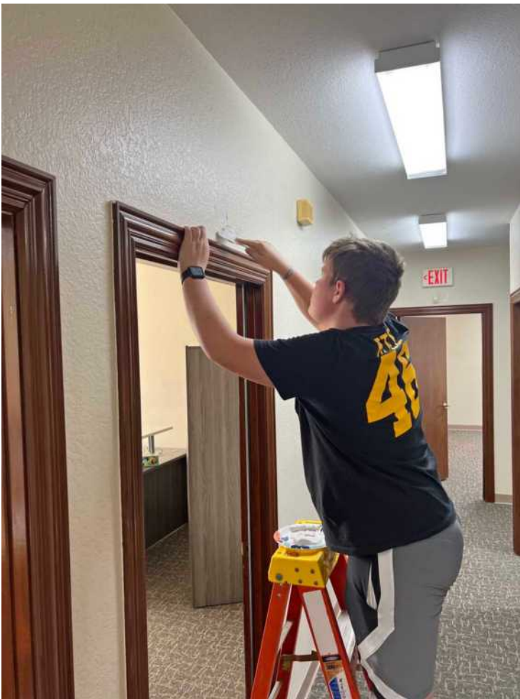
Carver Ede, son of Pastor Tony D. Ede, filling holes in the walls of the hallway of the new NALC offices. His brother Liam also helped with the repairs.
